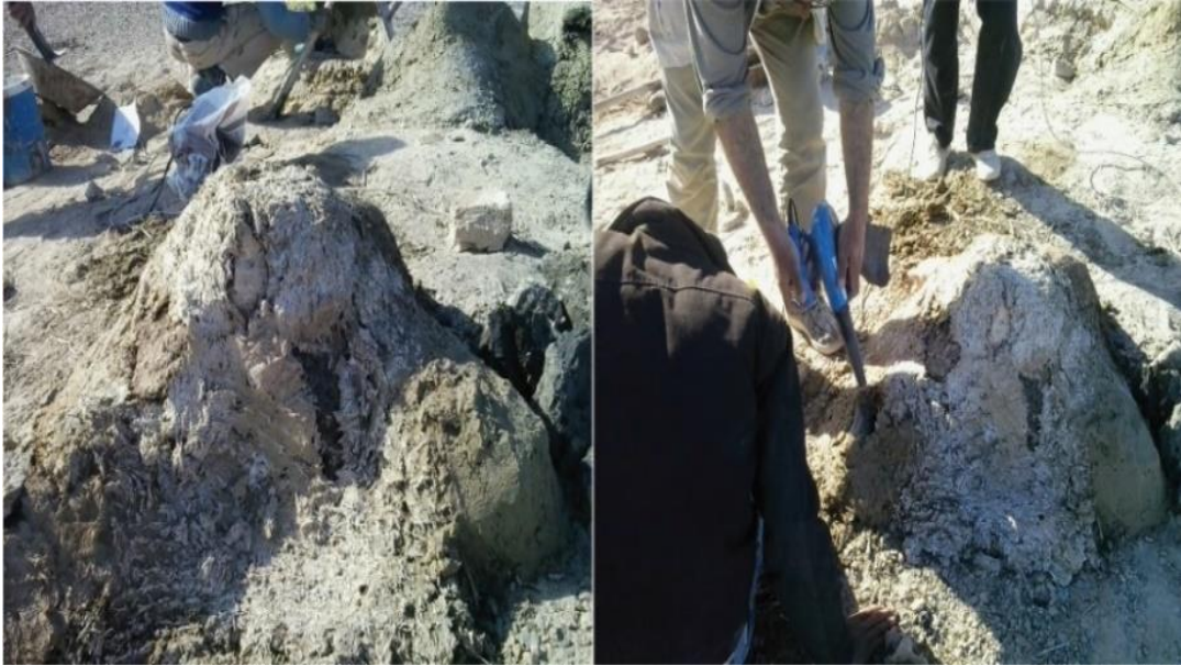
Figure 14: Kiln No. 2, constructed with a domed roof and a deep in-ground reservoir. Electric Blower was created using a blower to increase temperature for pottery firing. A thermocouple was installed to measure the temperature, but measurement was ultimately halted due to generator fuel depletion (After: Mortazavi, 2015).
